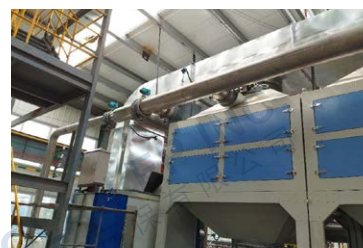
Start-up:2021 Industry:Metal smelting Volume:40000Nm 3 /h
