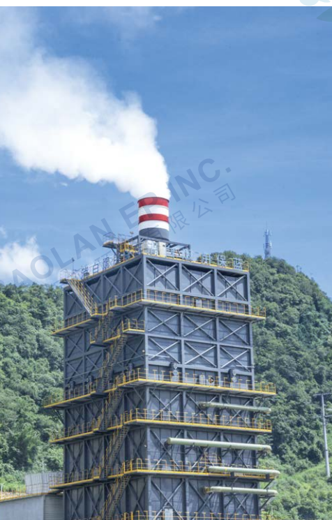
Prior to Equipment Startup
