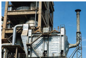
Start-up:2024 Industry:Iron and steel Volume:180000Nm 3 /h
