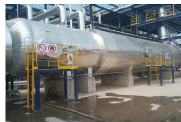
Start-up:2025 Industry:Coating Volume:8000Nm 3 /h
