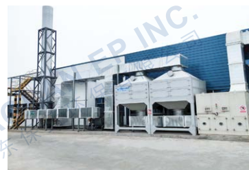
Start-up:2020 Industry:Electronic equipment Volume:40000Nm 3 /h
