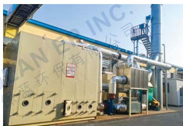
Start-up:2019 Industry:Chemical materials Volume:30000Nm 3 /h
