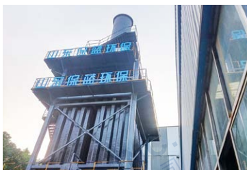
Start-up:2021 Industry:Steel Volume:150000Nm 3 /h
